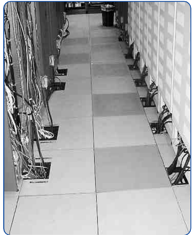
This hot aisle on the discharge side of IT equipment should literally be hot. Perforated tiles improperly placed in the hot aisle reduce cooling effectiveness.
